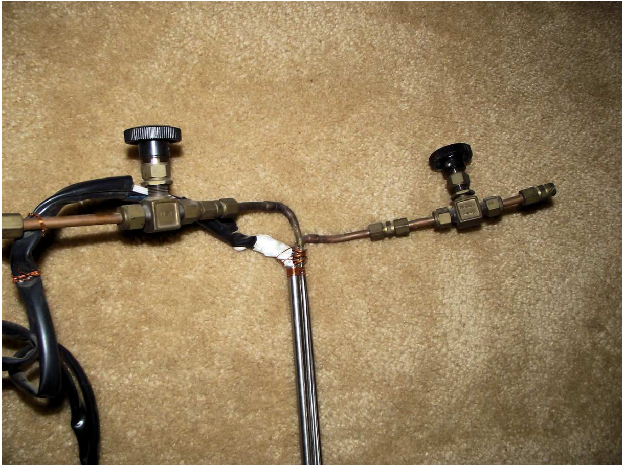
Figure 14. QMSD Unit's Gas Supply Lines with Inlet and Outlet Valves and Electrical Wiring
