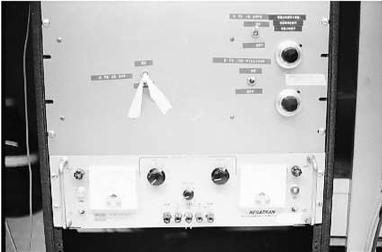
Figure 29. Photo of Rack-mounted Regatran 0-120-amp Power Supply with two 10-turn Potentiometers
